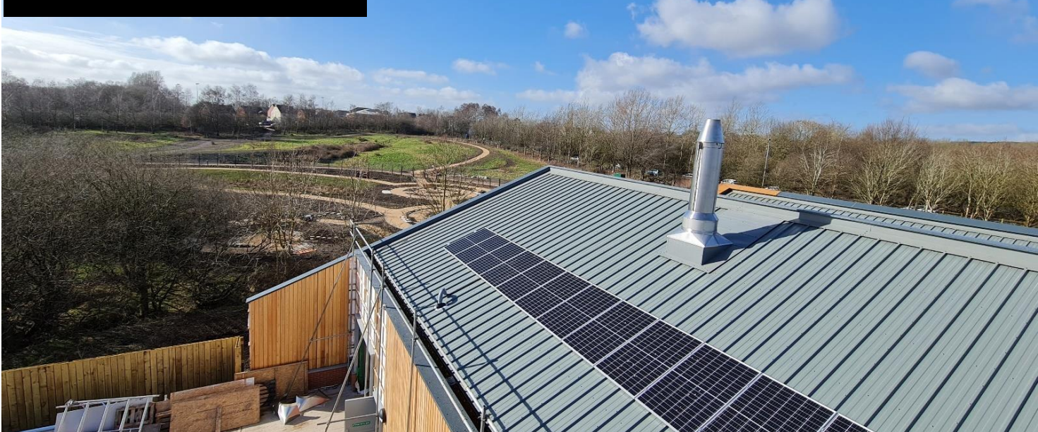
Photo: Solar PV, Cannock Chase
